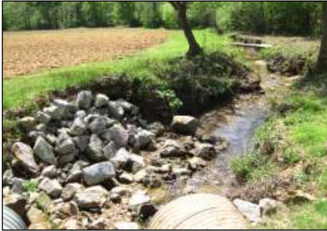
Channel and bank erosion
