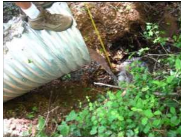
Poor crossing fill condition
